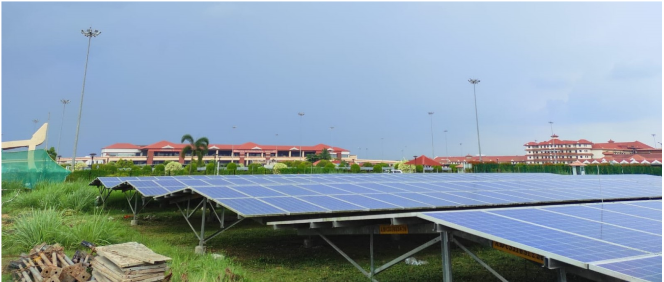
Solar farm at Kochi International Airport
